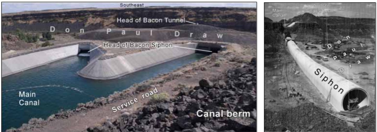
Figure 6. Head of the dual Bacon Siphon and Tunnel of the Columbia Basin Project. Left: Irrigation water in the Main Canal splits into two conduits before disappearing into the Bacon Siphons. Looking south. Right: Construction of the 1,000-foot-long siphon (now buried) spans Don Paul Draw, circa 1946, looking north. Photo courtesy of Central Washington University Archives, Rufus Woods Photographic Collection. A second buried siphon leading to a parallel tunnel was completed in 1980.
